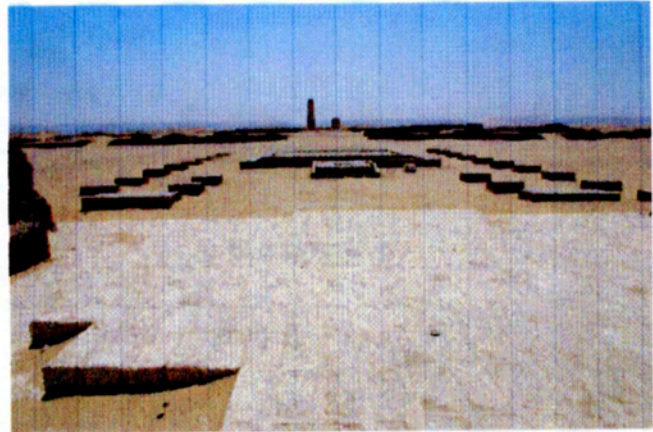
Conservation at the Small Aten Temple. General view to the east, along the main axis, of the work completed so far.
