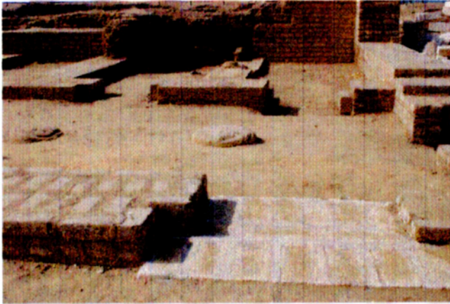
Work begun in 2005 at the North Palace. Repairs to the domestic suite, including the bathroom. View to the south. The remaining step is to replace the stone bathroom floor that was present in 1923 but has since vanished.
